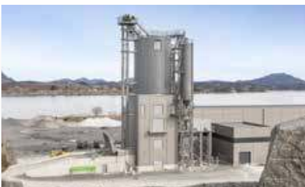
Batching and mixing plants
