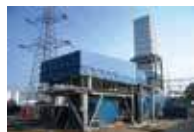
GAS TURBINE POWER PLANT
