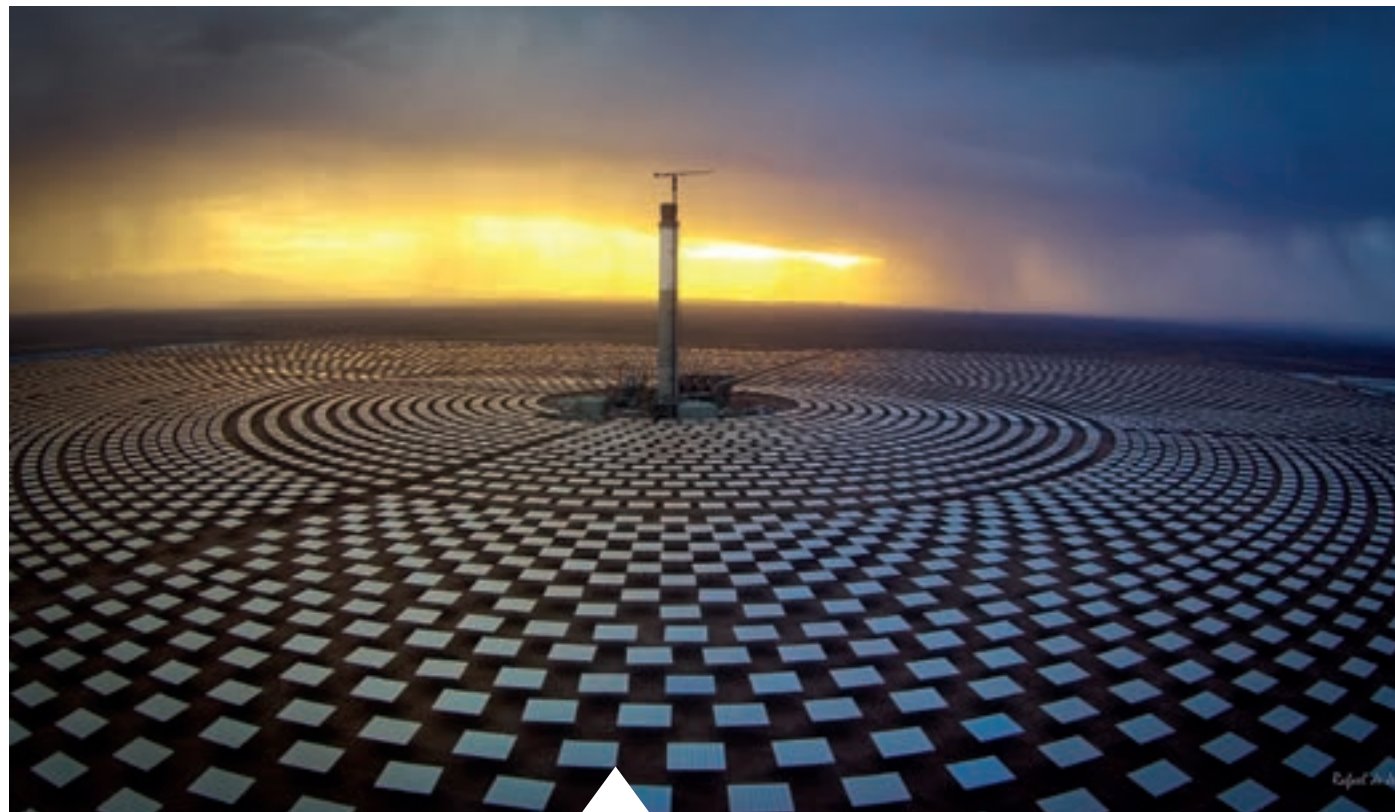
Planta solar termoelectrica Noor III / Noor III solar thermal power plant.
