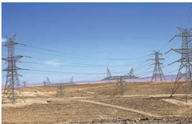
400 kV Al Qatrana-New Ma'an Transmission Line, Jordan
