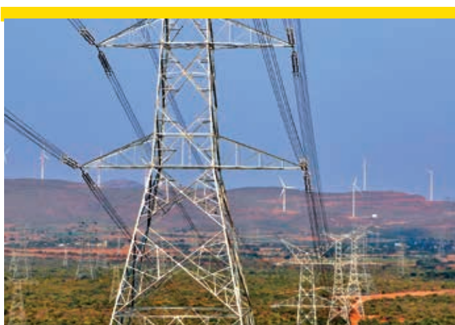
765 kV Chilakaluripet-Cuddapah Vemagiri Transmission Line, Andhra Pradesh
