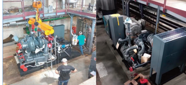
Installation of BP compressors at Fauga Mauzac
