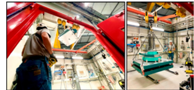
Installation at SpLine of equipment for single-crystal characterisation by X-ray diffraction.
