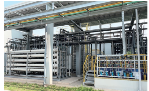
Water recycling facilities (YKK Vietnam Co., Ltd. Dong Van Factory)
